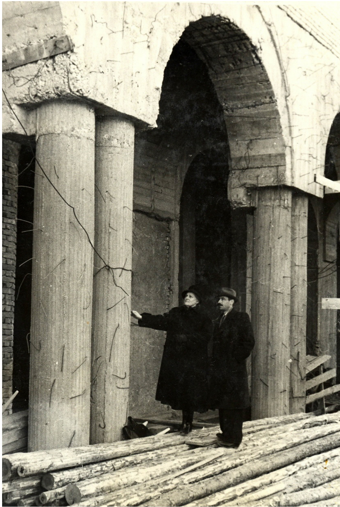
Construction site of the House of Academics, with architect Ketevan Sokolova-Qurdiani (1905-1988), first women architect in Georgia
